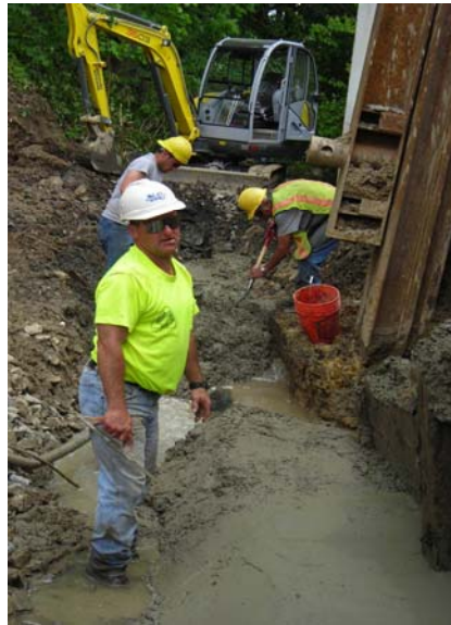
Dan Galetti, John Duda, and George "JR" Parsons install concrete around 18" CIP at Willow Grove on May 26, 2009.
