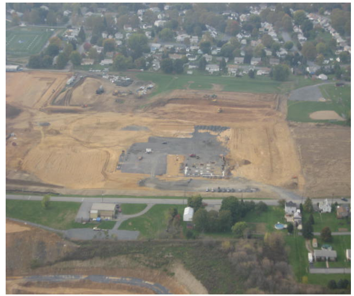
Aerial view of Nazareth Middle School courtesy of Joe Horton, Penn Builders.
