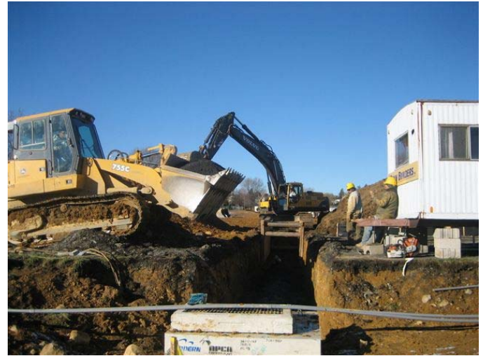
Matthew Chapman's crew installing 42" storm pipe at Nazareth Middle School. Dennis Snyder, Chad Ulrich, Jason Udit, and Brian Jesse.
